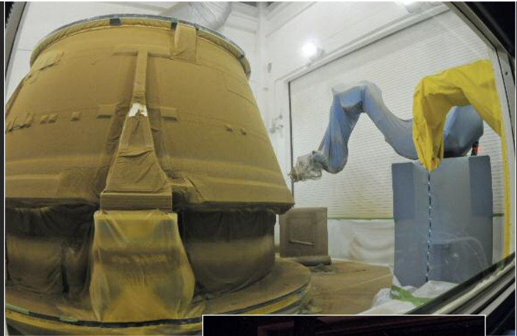
An SRB aft skirt receives a robotically controlled layer of Marshall Convergent Coating-1 Thermal Protection System material.
