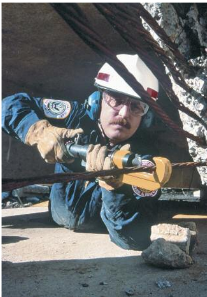
NASA-developed tool, licensed under the name "LifeShear," used at the bombed Alfred P. Murrah Federal Building (1995), Oklahoma City, Oklahoma.
