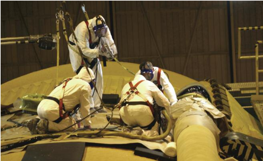
In what used to be a one-person operation, a team of technicians at NASA's Michoud Assembly Facility prepares to hand-spray BX-250 foam on the bipod attach fittings. The videographer (standing) records the process for later review and verification. A quality control specialist (left) witnesses the operation, while two spray technicians make preparations.
